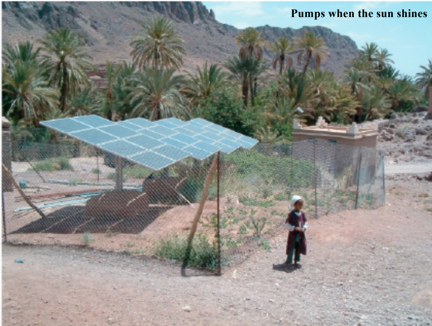
Figure 5.2 Off the grid: PV water pumping for a Moroccan village (EPIA/Isofoton).
