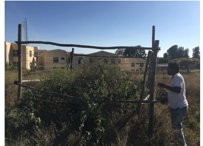
Well and Solar Pump
