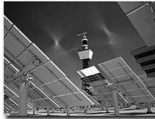
FIGURE 10.7 Heliostat detail of the Solar Two plant (source: www.energylan.sandia.gov/sunlab/overview.htm ).
