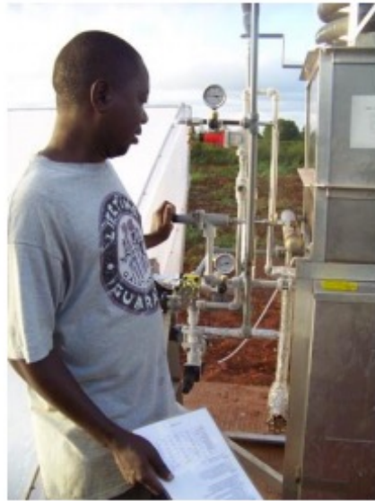
Figure 11. The system is operated by manual valves. Operation is routine and easy to do. The valves are operated in the morning and late afternoon. Water to be frozen is put into the evaporator in the afternoon; it is ready to be removed as ice early the next morning.
