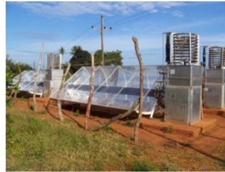
Figure 3. Three units were installed in Kilifi District at Sovimwamri Dairy.
